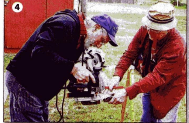
>> PHOTOS: JAMES DUDLEY 1) Construction progresses as many work; 2) Reita Barnes works on a quilt bag; 3) Pastor Jerry Graves visits with Bob Martin; 4) Jack Hawken and Harold Poling trim the edge of a sheet of siding.
